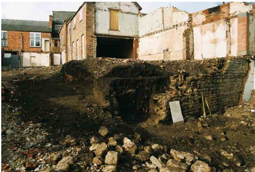
Plate 6 General view looking northwest showing position of terrace and wall to rear of buildings.
