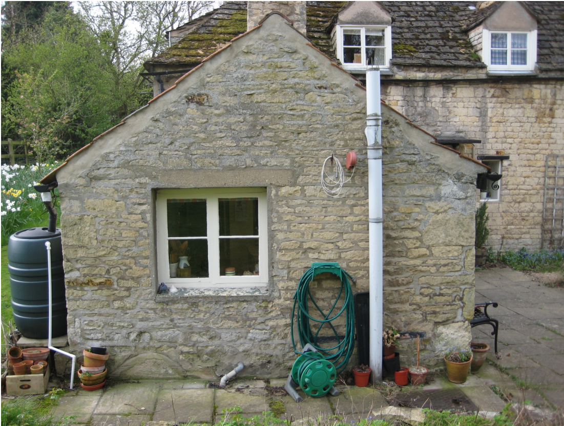
Plate 1 Detail of north elevation of north wall of kitchen wing to be altered by extension, looking south
