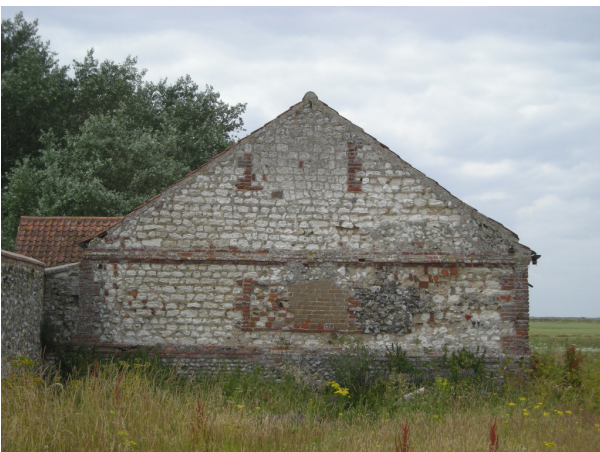
Plate 3 – The east end of the threshing barn showing blocked openings, looking west
