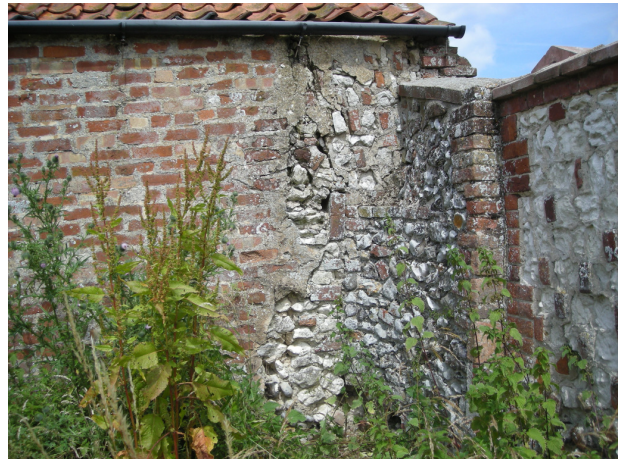
Plate 5 – Ragged join at southeast corner of the barn, looking northeast
