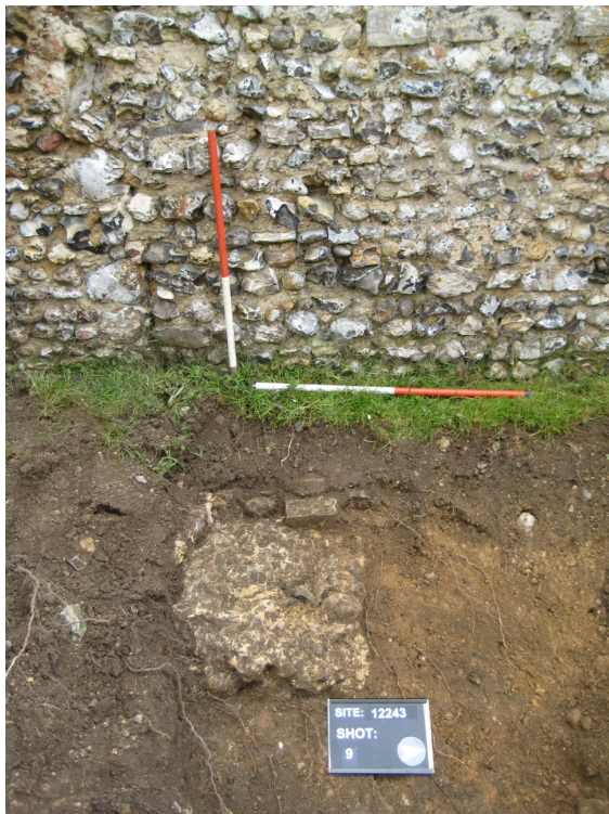
Plate 4 South facing view wall (001) showing alterations to flint work in the north nave wall
