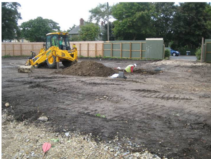
Plate 6 Southwest facing view of site, looking towards Newport showing Trench 3 under excavation
