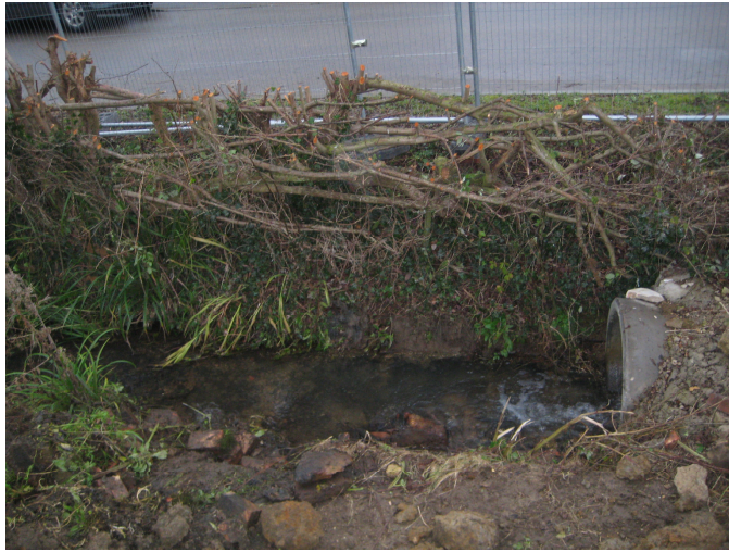
Plate 4 Modern culverted line of stream along northern property boundary showing force of modern flow
