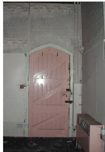
Plate 12 Door in southwestern corner of nave, showing brick arch over, looking south
