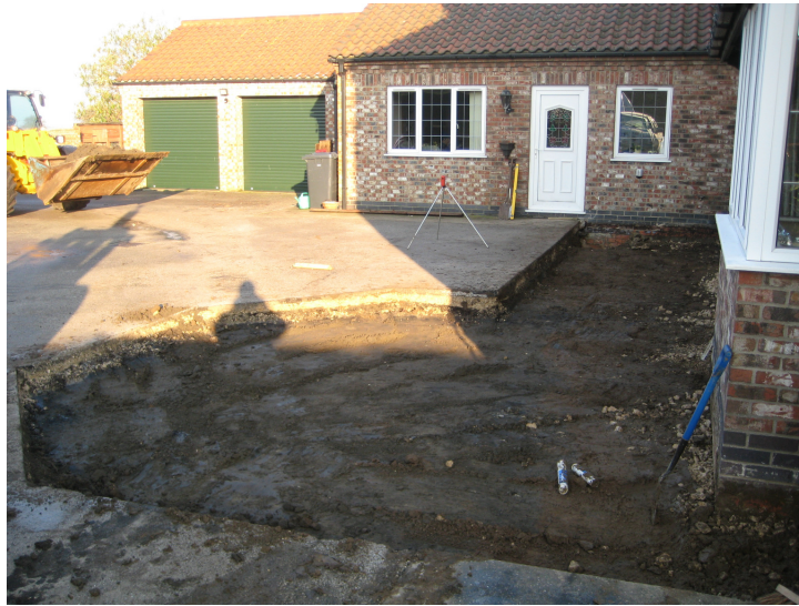
Plate 1 – View showing the stripped area prior to the excavation of foundation trenches, looking north
