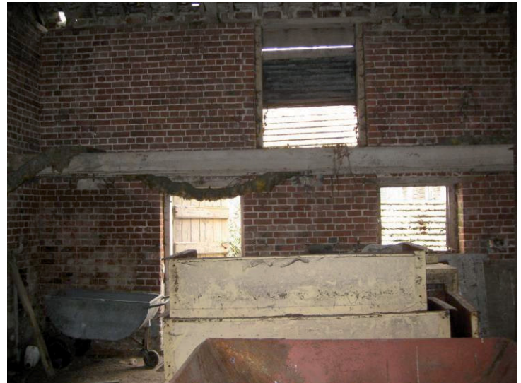
Plate 23 Northern elevation inside west room of main barn and surviving joists of upper floor, looking north
