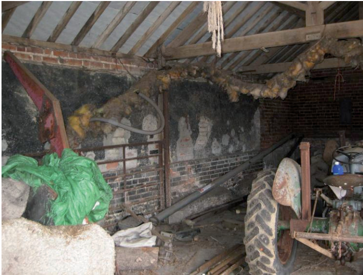
Plate 12 Northern room of western animal accommodation range, general internal view, looking northwest
