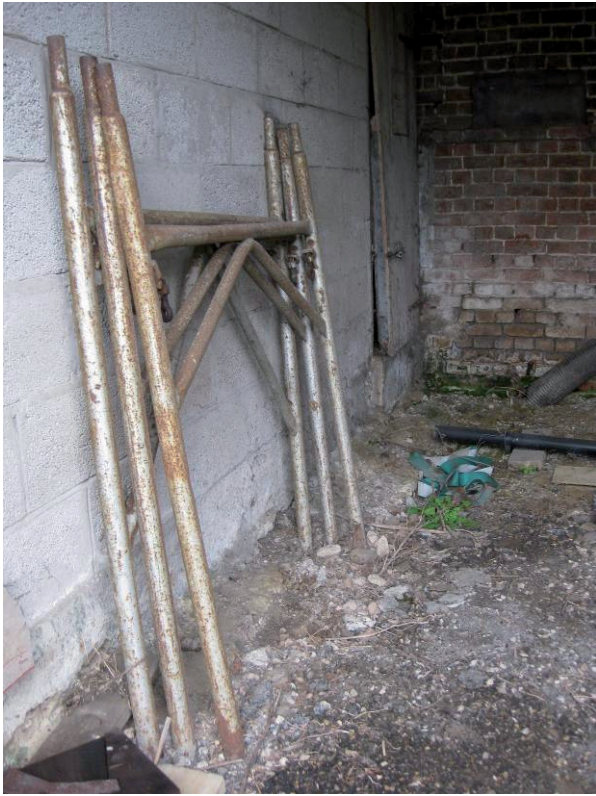
Plate 15 Dividing wall between western and northwestern ranges, internal, showing breeze block construction over unfired clay block, looking north
