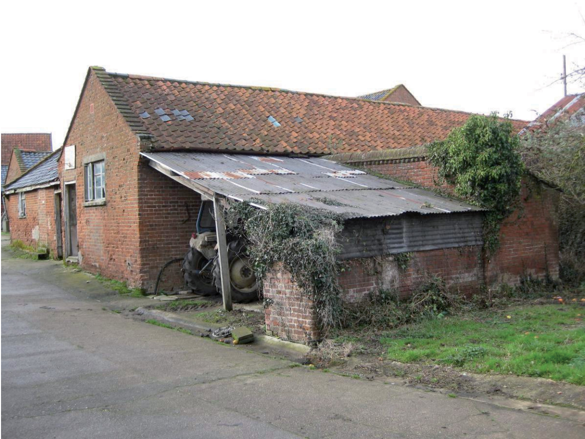
Plate 34 General view of buildings showing east and south walls of eastern range of animal accommodation, south wall of east-west range and lean-to shelter, looking northwest
