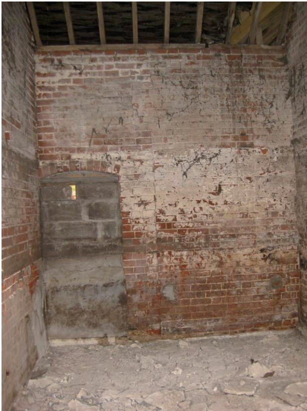
Plate 5 Southern stable or loose box at north of cart shed, west wall internal showing blocked doorway and straight join, looking west
