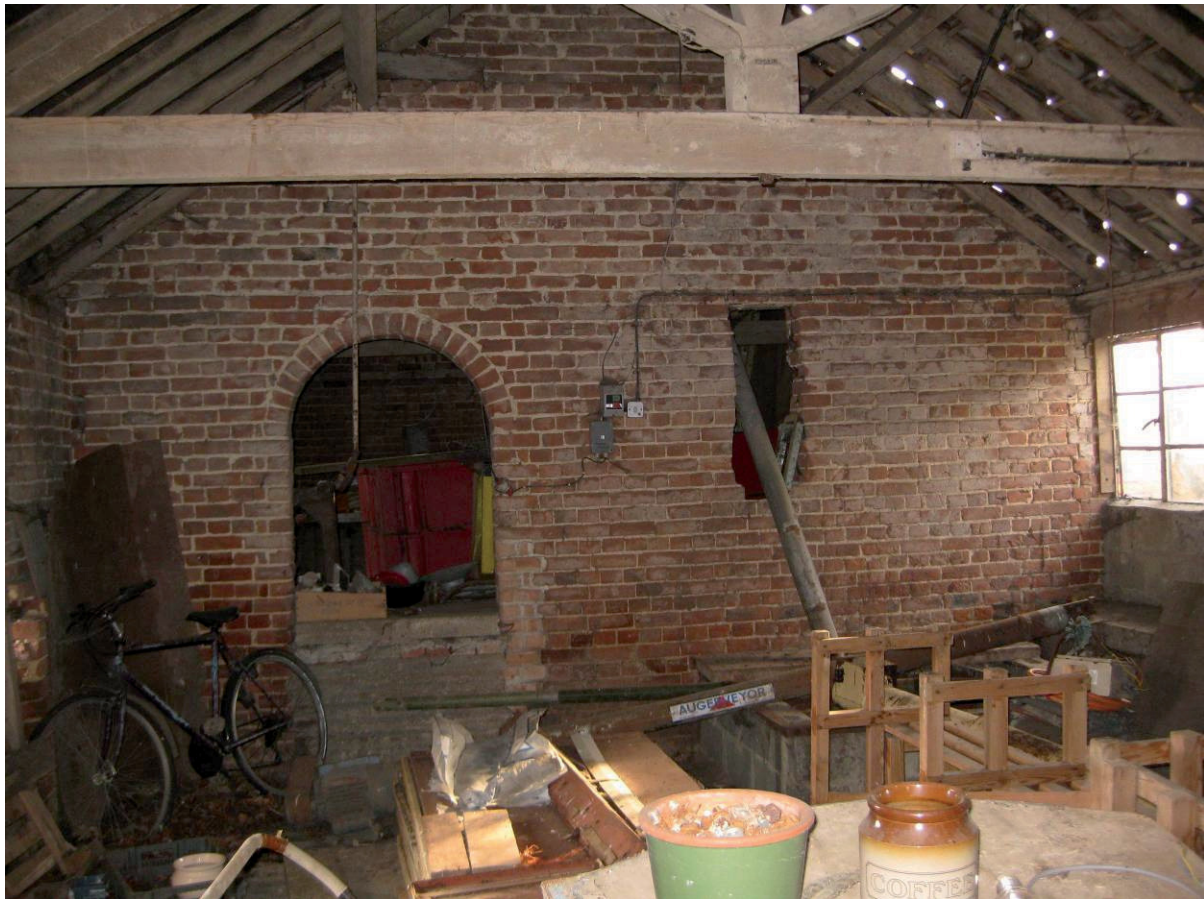
Plate 37 Central dividing wall inside north-south range, possibly for fodder storage, showing partly blocked doorway and inserted opening, looking south
