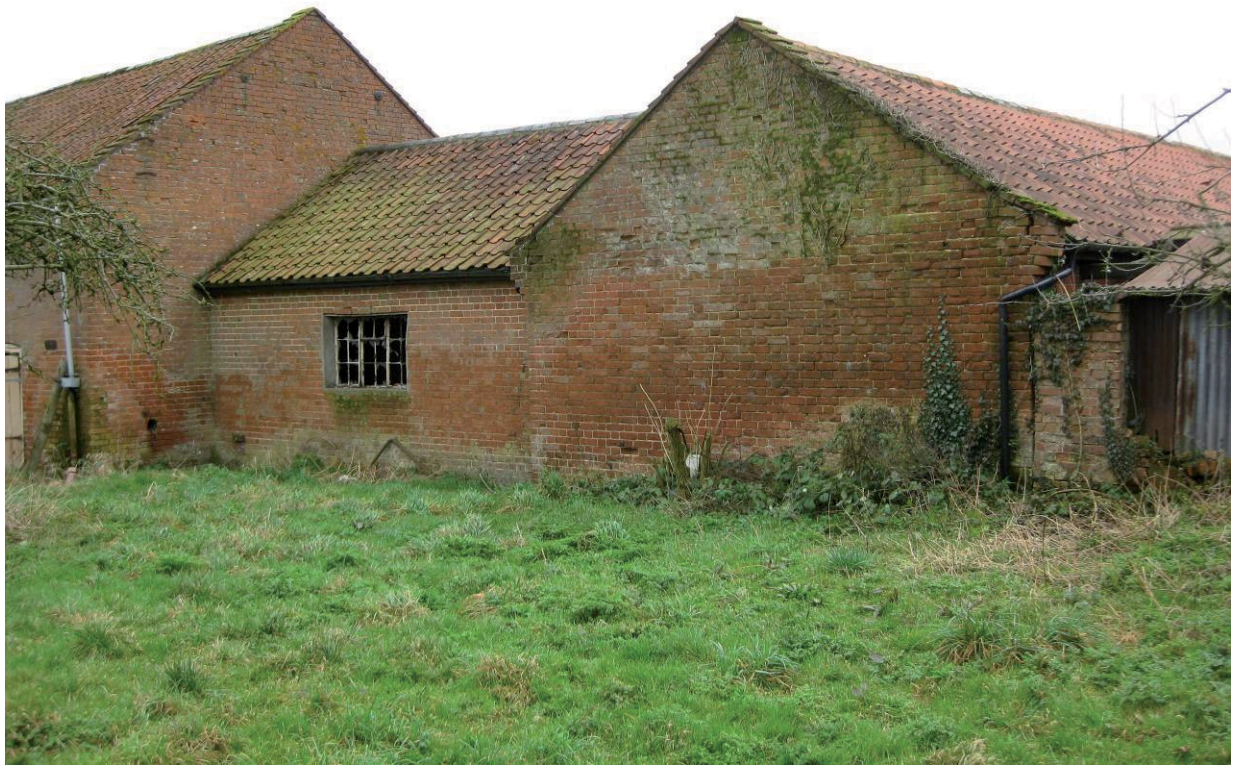
Plate 18 Exterior view of northern walls of westerly and northwesterly ranges of animal accommodation and main barn, looking southeast
