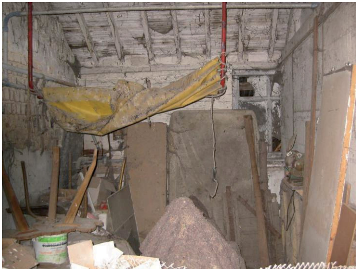
Plate 35 Interior of southern room of eastern range, showing breeze block partition wall, looking east
