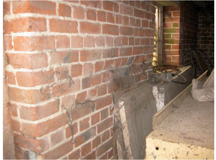
Plate 22 Detail of walling, northern wall inside west room of main barn, showing wear pattern of bricks, perhaps due to machinery, looking northeast
