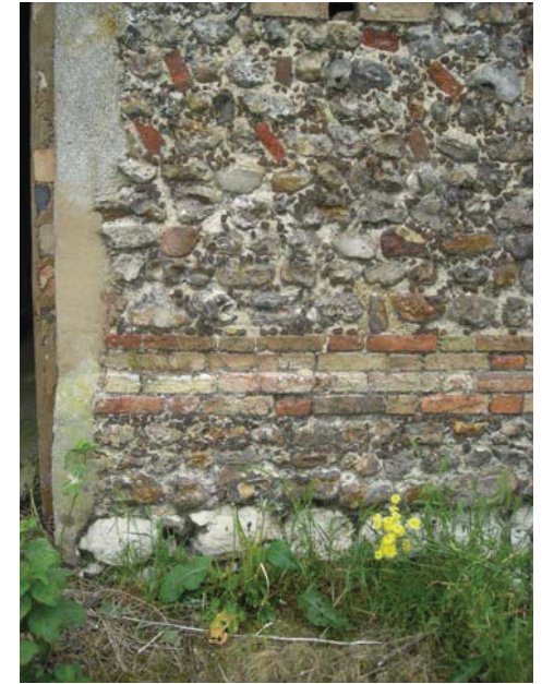
Plate 11 Detail showing construction of north gable end of main barn, looking south
