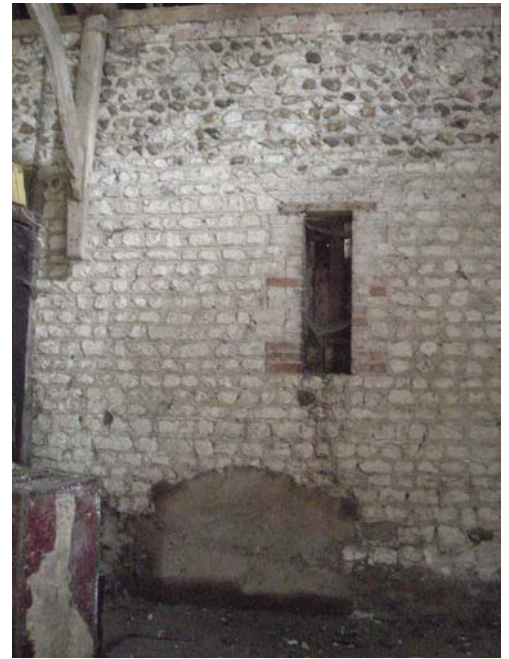
Plate 14, Interior of main barn, showing breather slit and low blocked opening, looking west
