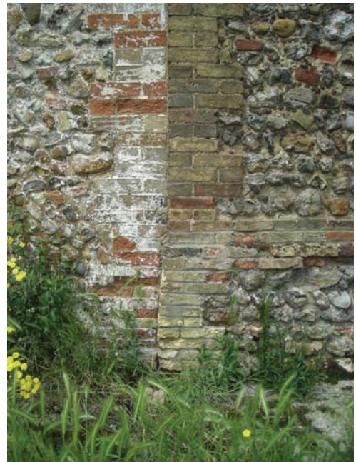
Plate 7 Detail of walling and join between main barn (at right) and adjacent building (at left), east elevation, looking west
