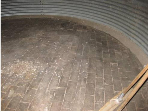
Plate 16 Interior of main barn, brick flooring in western bay (inside silo), looking west.
