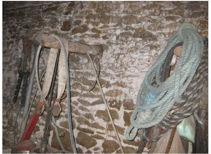
Plate 28 Detail of wooden tack pegs in north wall of tack room, looking northwest
