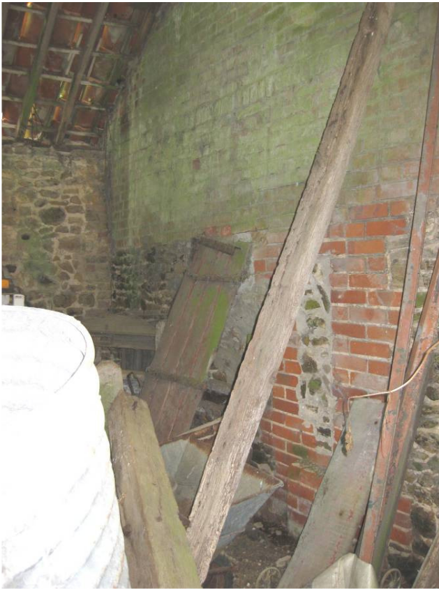
Plate 39 Cartshed interior showing south gable end with 20 th century brickwork above eaves level, looking southeast.
