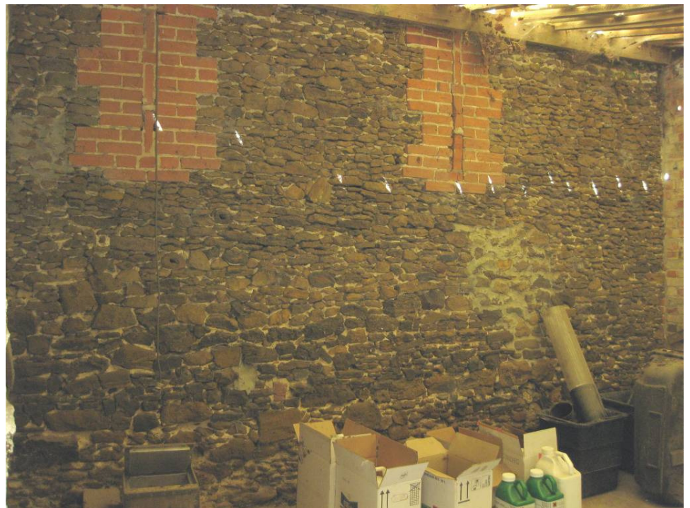
Plate 12 Lower part of east gable end of main barn as seen from interior of chemical store. Note blocked breather slits, looking northwest.
