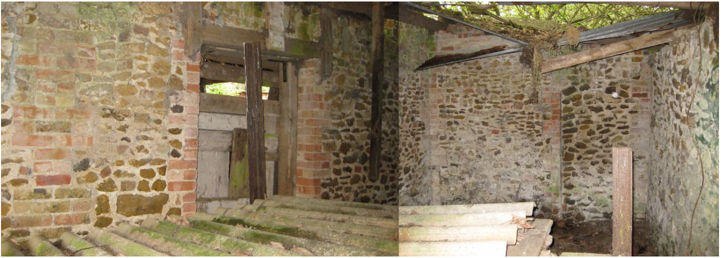
Plate 35 Interior of store 1 showing detail of door in south wall and quoins in west wall, looking southwest and west.
