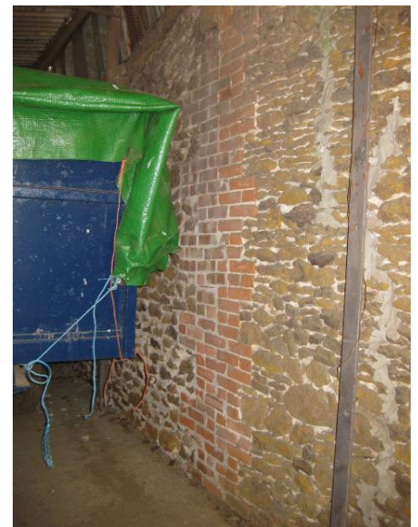
Plate 7 Detail of northeast corner of northern wall of main barn at join with north wall of chemical store, looking southeast.
