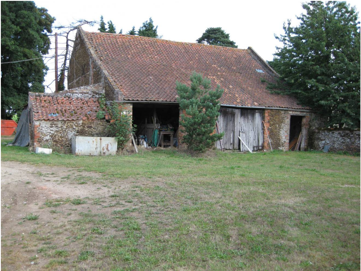
Plate 8 View of main barn from south showing catslide roof over stable 1, barn porch and stable/loose box 2. Tack room at far left (looking northeast).
