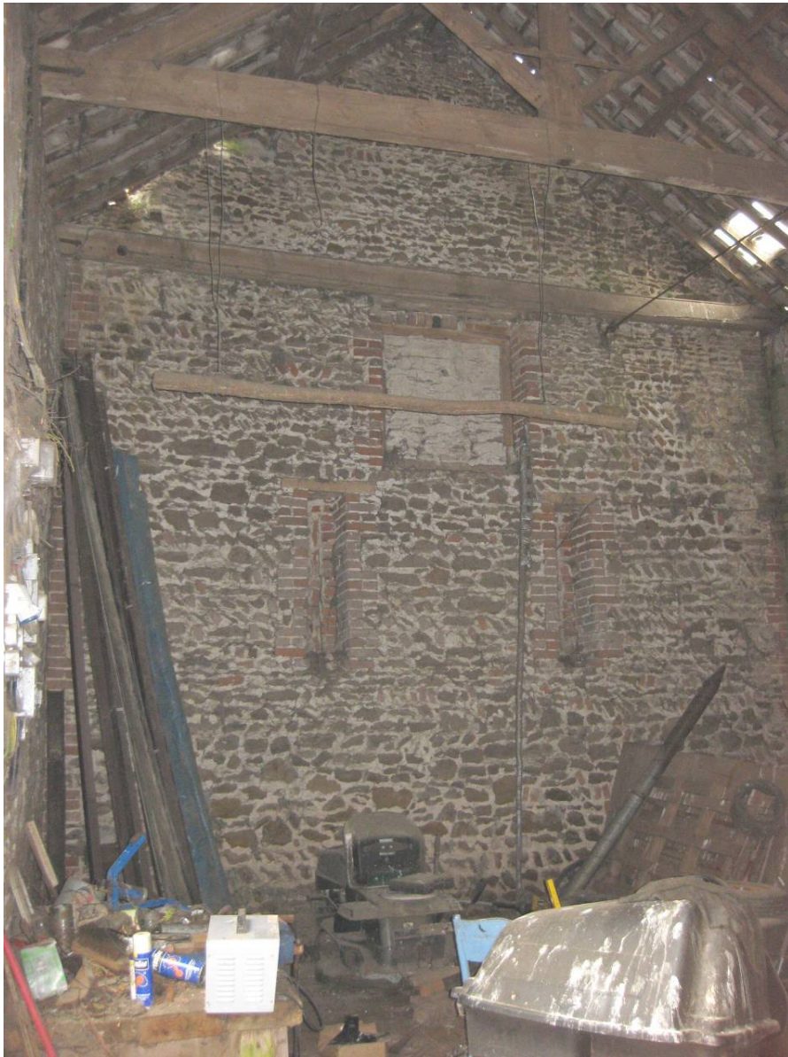
Plate 13 East gable end of main barn from interior of barn. Note blocked pitching hole and breather slits, looking east.
