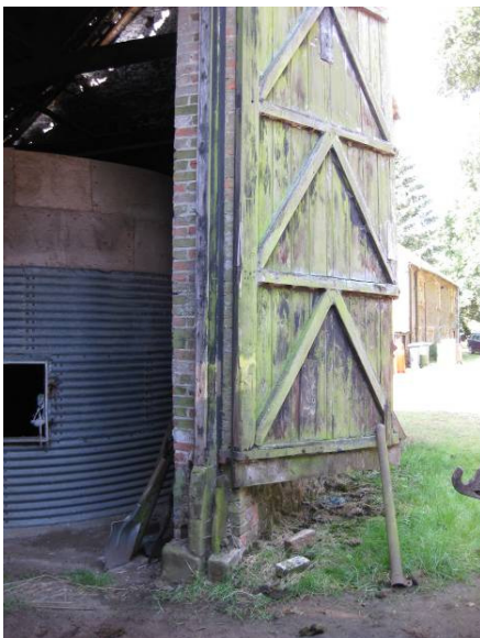
Plate 5 Wooden door of northern wall of main barn. Possibly an original feature, note gap at base of door, looking west.
