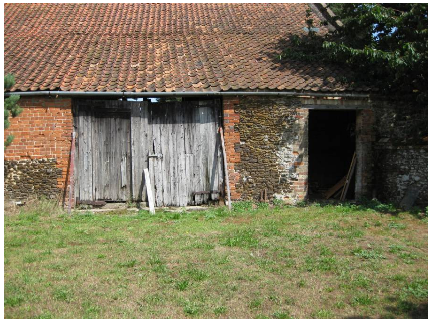
Plate 10 Detail of paired wooden doors of barn porch and entrance to stable/loose box 2 at right, looking north.
