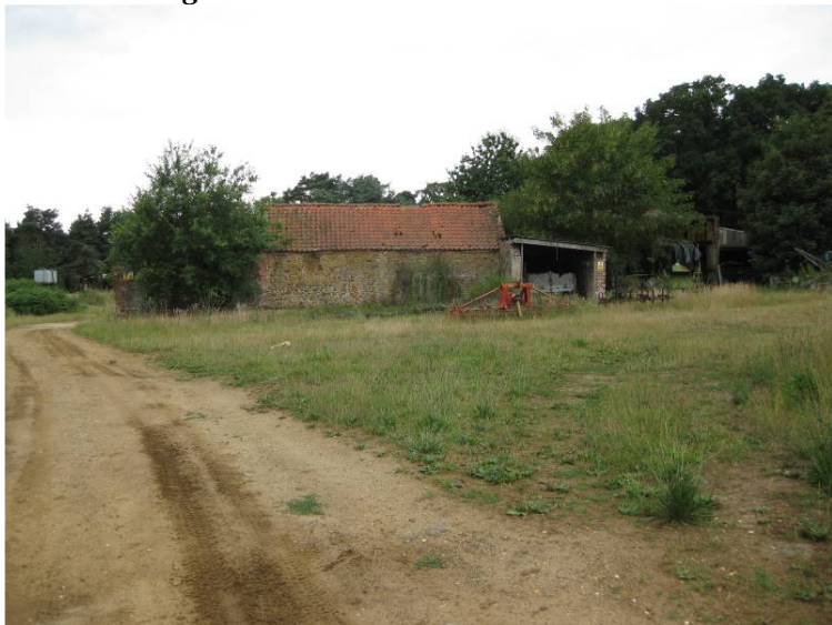
Plate 31 General view of eastern range, rear of cart shed at centre, looking west
