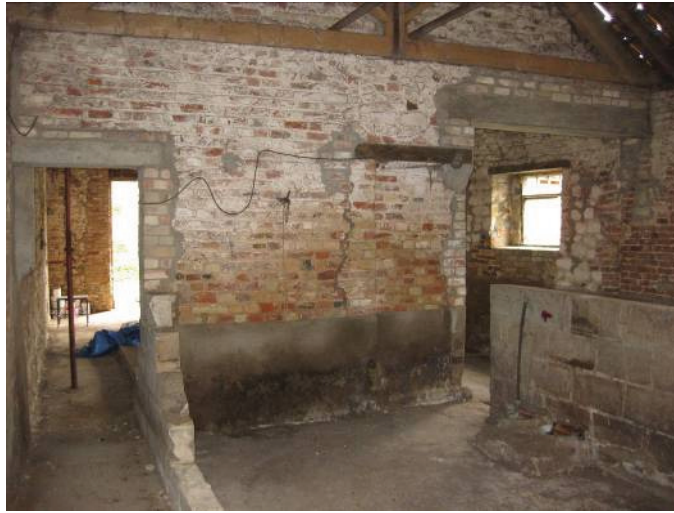
Plate 52 - Interior of Room S, showing modern breeze block animal pens, late 18 th century or earlier dividing wall with probable 19 th century doorway, subsequently blocked, and modern openings, looking northwest
