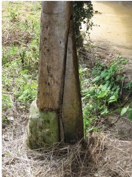
Plate 41 - Detail of original 19 th century timber stanchion and stone stanchion base of open-fronted shelter T, looking southwest
