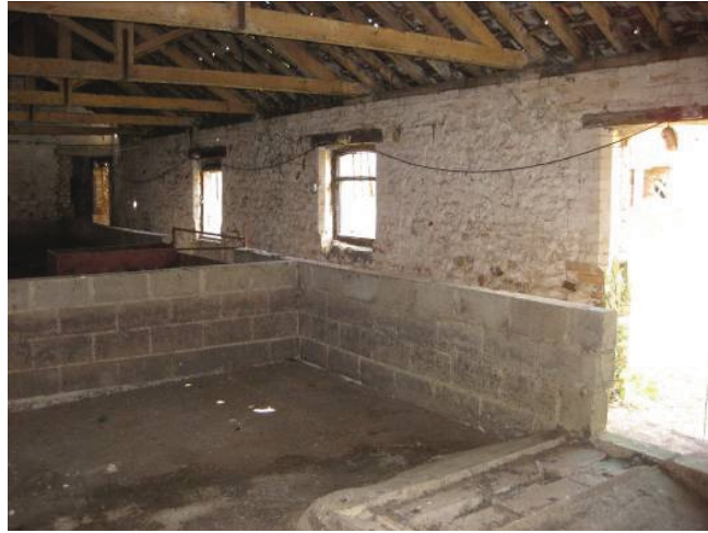
Plate 43 - Interior of Room L showing original doorways and windows and modern breeze block animal pens, looking northwest
