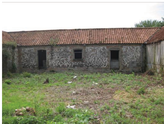
Plate 42 - Northern wall of Room L, viewed from Yard 4, showing 19 th century walling, window opening and doorways, one recently partially blocked, looking south
