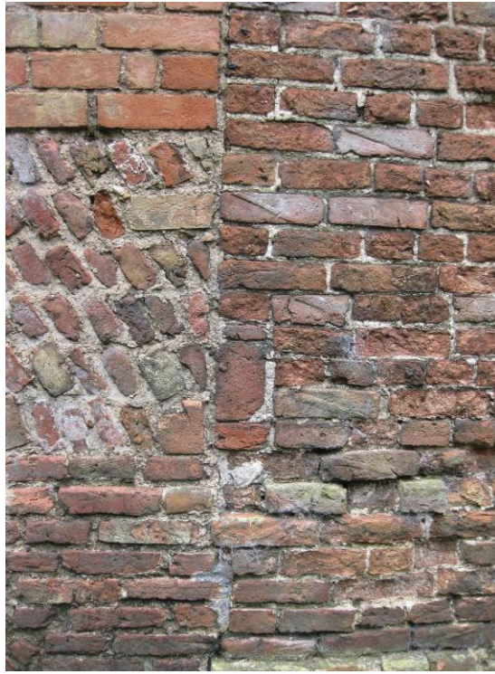
Plate 57 - Detail of northern wall of Room S showing join in walling, 19 th century bricks evident at top left, and late 18 th century or earlier bricks below and to right, some with clear diagonal skintling marks, looking south
