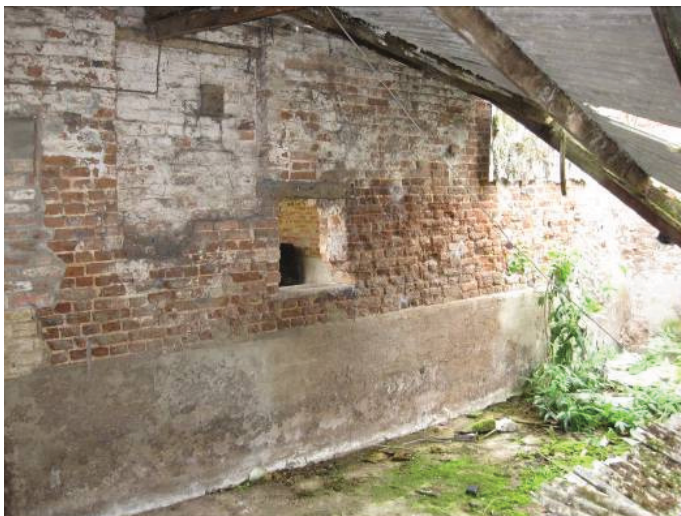
Plate 54 - Detail of southern wall of Room S showing late 18 th century or earlier walling, blocked opening and possibly inserted opening, looking northwest
