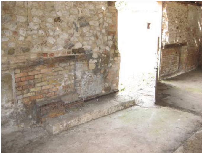
Plate 32 - Detail of western wall of Room P, showing recently widened central doorway and infilled low openings, probably 19 th century openings for pigs or similarly-sized animals, looking north
