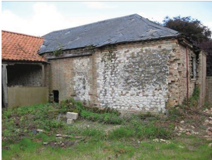
Plate 20 - Rear of Room J, showing collapse and 20 th century repairs to southern elevation, 19 th century doorway for sliding door with modern infill and insertion of smaller opening for pigs or similarly-sized animals, looking east
