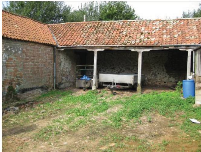
Plate 23 - Open sided shelter K and 20 th century walling at western end of building I, viewed from Yard 3, looking west
