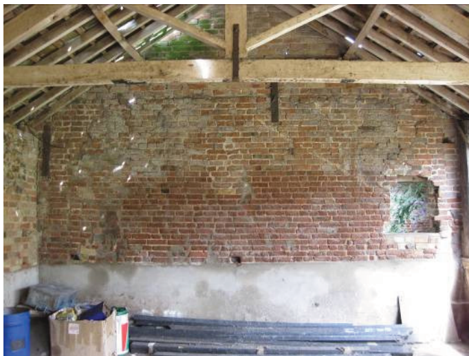
Plate 48 - Western wall of Room S as viewed from interior of open-fronted shelter T, including late 18 th century or earlier brickwork, looking north
