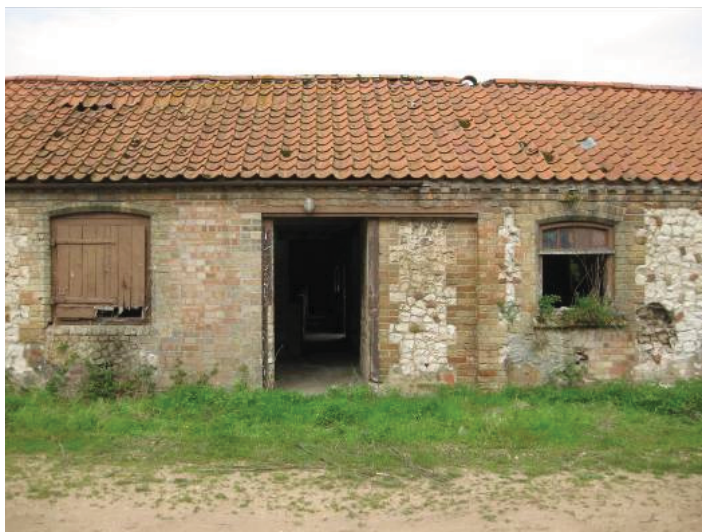
Plate 30 - Frontage of Rooms O and P, showing shuttered window and sliding door to Room O and half-glazed window to Room P, looking west
