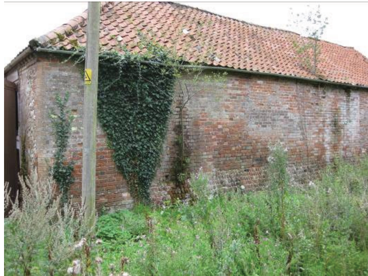
Plate 56 - Northern wall of Room S, showing 20 th century repair at left and late 18 th century or earlier walling at right, looking southwest
