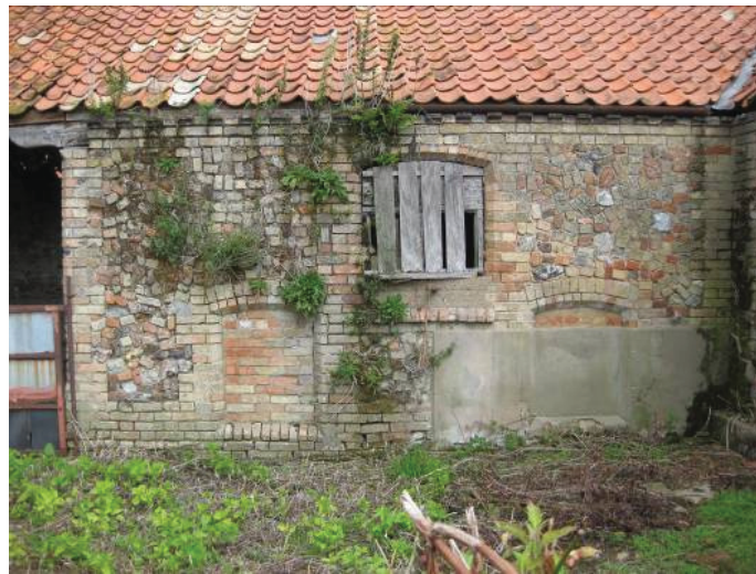
Plate 8 - Exterior of Room C from Yard 1, showing blocked low openings and half-glazed window, looking north
