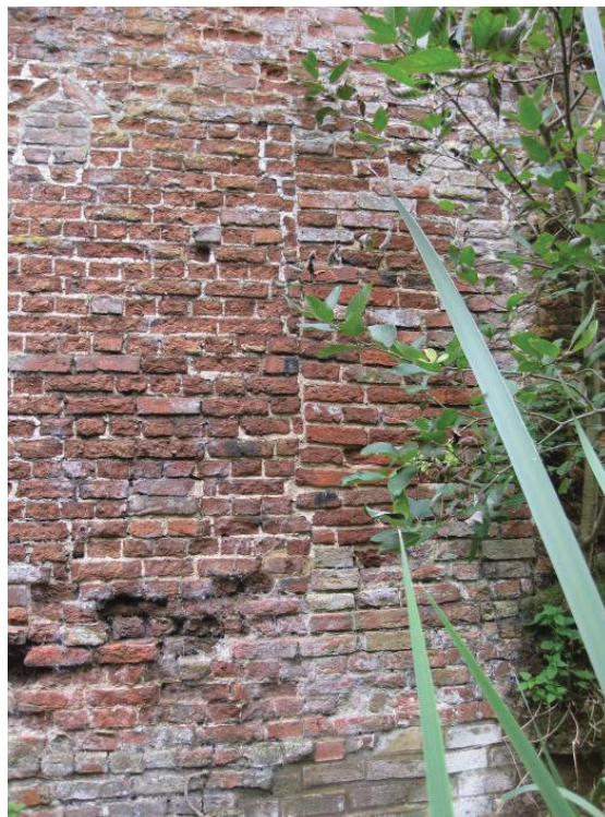
Plate 58 - Detail of northern wall of Room S showing right edge of infilled opening and smaller blocked opening within this infill, all of late 18 th century or earlier brick, looking south
