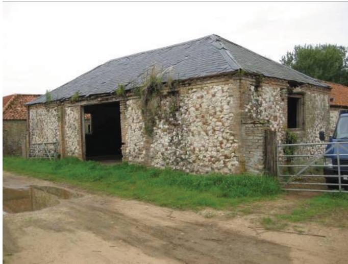
Plate 19 - Frontage of Room J, showing large double doorway, the roof of this building having been replaced by slate, looking southwest
