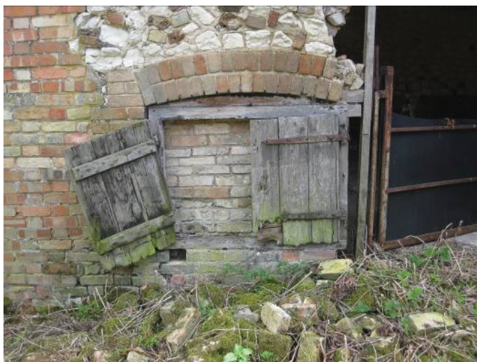
Plate 36 - Detail of blocked opening to Room P, showing probable 19 th century brickwork surround and shuttering, looking east
