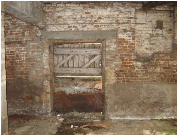
Plate 53 - Detail of southern wall of Room S showing elements of late 18 th century or earlier walling and stable door of possible 19 th century date
