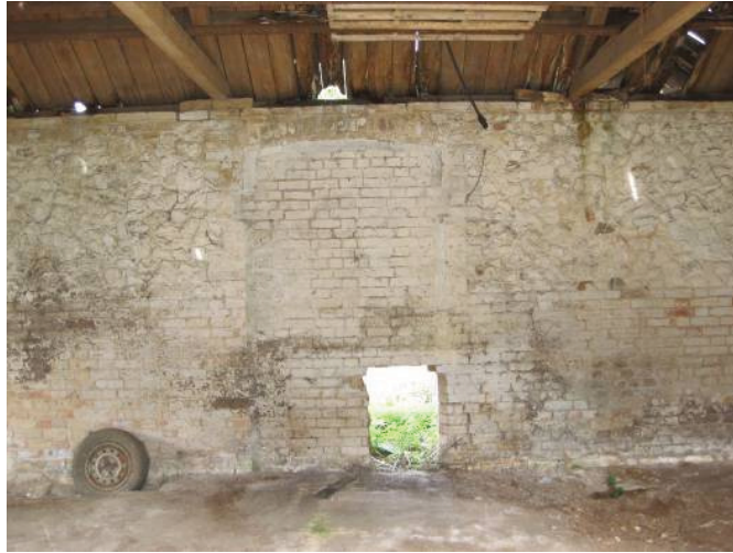
Plate 22 - Blocked doorway and inserted small opening in western wall of Room J, looking west
