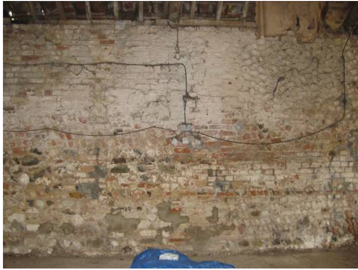
Plate 55 - Detail of northern wall of Room S showing variation and patching of 18 th , 19 th and 20 th century date, looking north
