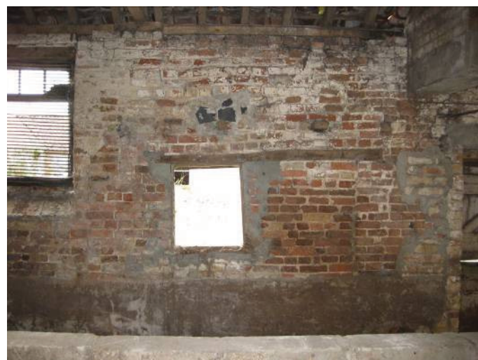
Plate 51 - Detail of southern wall of Room S showing openings including possible 19 th century window at left, probable late 18 th century or earlier brickwork, and blocked opening, looking south
