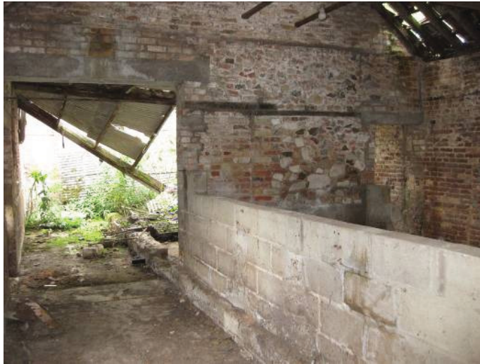
Plate 49 - Interior of Room S, showing modern breeze block animal pens, late 18 th century or earlier dividing wall with probable 19 th century doorway, subsequently blocked, and modern openings, looking northwest
