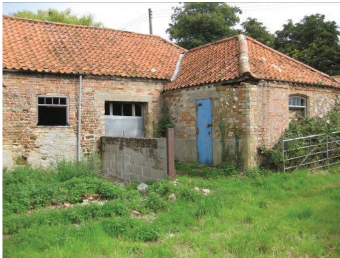
Plate 47 - Rooms S and R viewed from Yard 4, showing modern repairs to Room R, looking east
