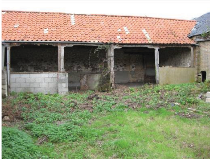
Plate 16 - Open-sided shelter I viewed from Yard 2, showing 19 th century timber stanchions and pillows infilled with modern breeze block, looking west
