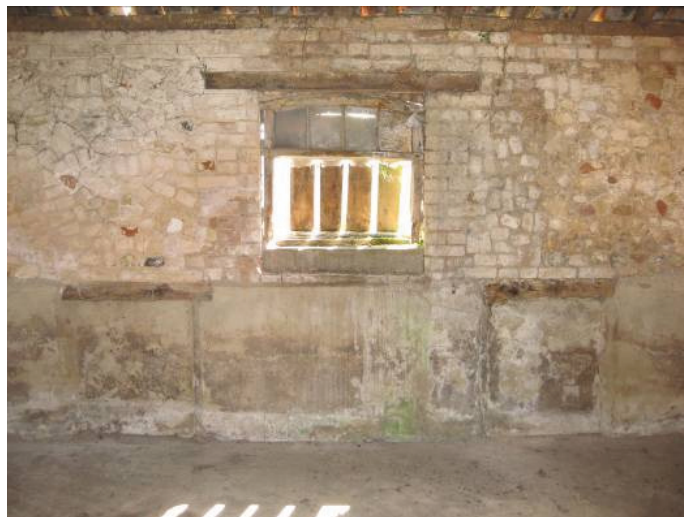
Plate 9 - Interior of Room C (reverse of wall shown in Plate 8), showing blocked low openings, looking south
