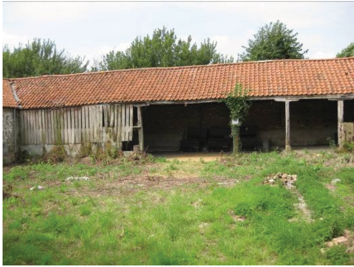
Plate 37 - Open-fronted shelter T at west of Yard 4, showing original 19 th century timber stanchions and pillars with modern infilling, looking west
