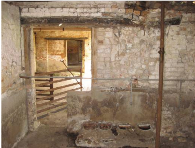
Plate 13 - Detail of doorway in Room E, showing probable 19 th century doorway for sliding door with modern alterations to create smaller opening for pigs or similarly-sized animals, view through doorway into open-sided shelter D, looking east
