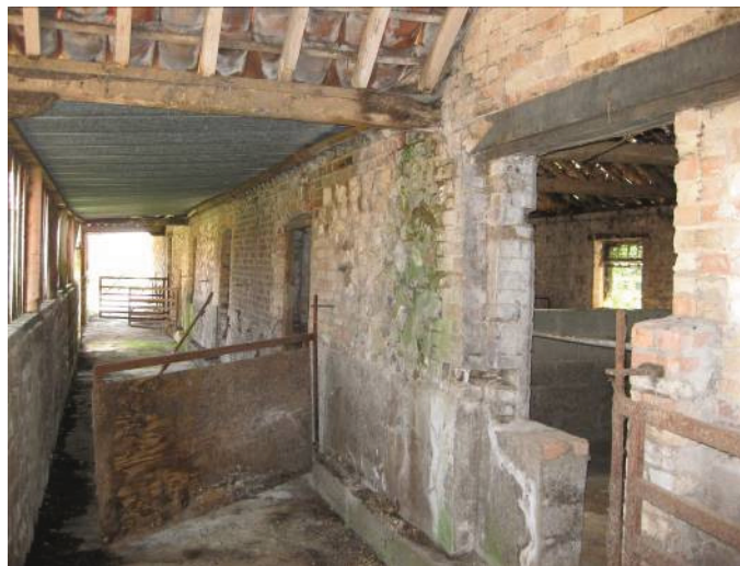
Plate 14 - Modern open-sided covered corridors H and F, showing 19 th century sliding doors of Rooms G and E altered to create smaller openings, and modern animal gates, looking south
