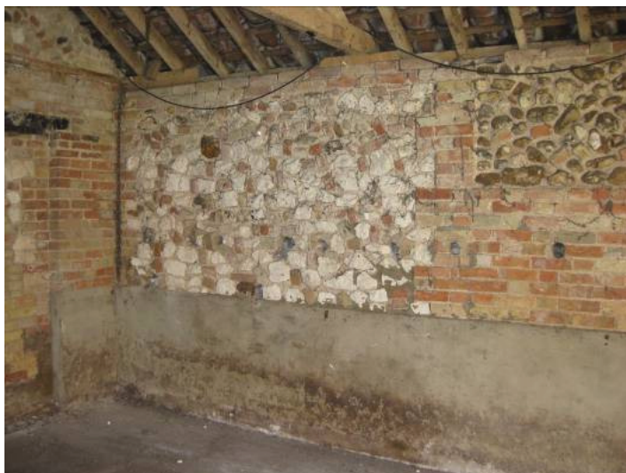
Plate 39 - Interior of open-fronted shelter T, showing series of holes in western wall possibly relating to former hay rack, looking southwest
