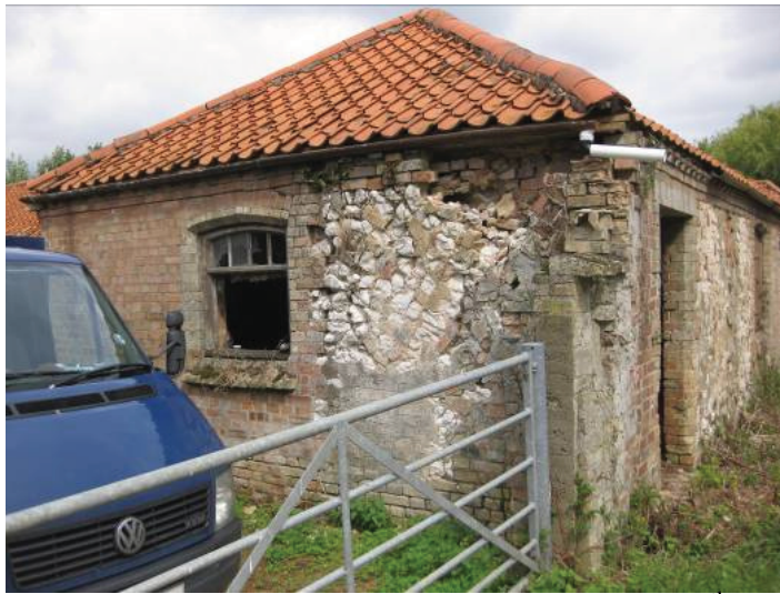
Plate 28 - Southern elevation of Room N, showing substantial 20 th century repairs and half-glazed window, looking north
