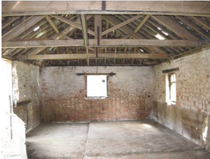
Plate 31 - Interior of Room P, showing 19 th century half glazed window at right, modern rebuilding of northern wall at centre and blocked low openings at left, looking north
