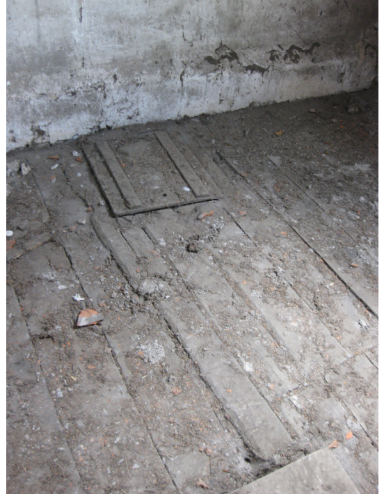
Plate 21 Upper storey, northern room, trapdoor and patched floor in southwestern part of room, looking west
