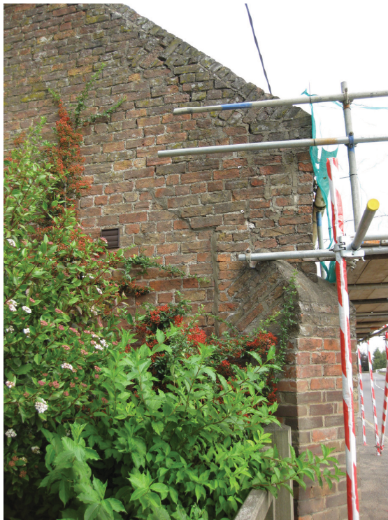
Plate 9 Southern elevation, east side, showing detail of straight joint, eaves scar and tumbling, looking northeast
