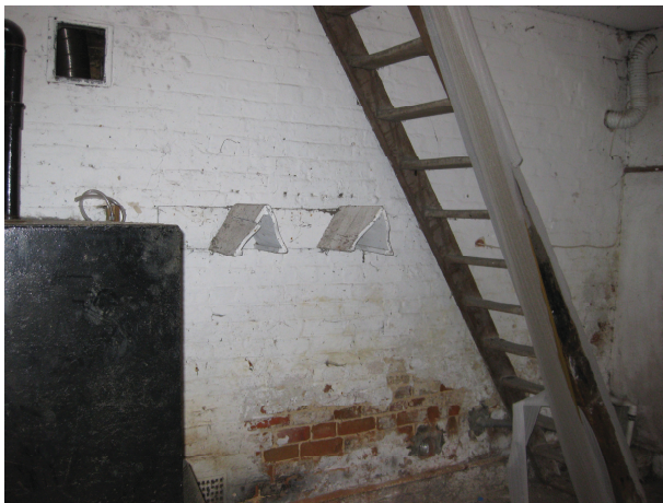
Plate 13 Ground floor, southern room, showing timber horse collar supports and stairs looking southwest
