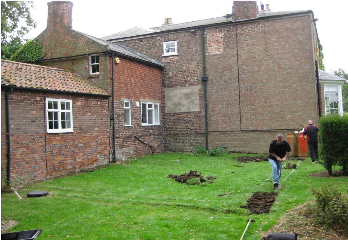
Plate 1 – General view looking south, showing removal of turf prior to digging footings
