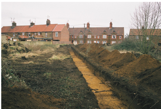
Plate 2 General view of the site from southeastern end of Trench 2 showing housing on Station Road, looking northwest
