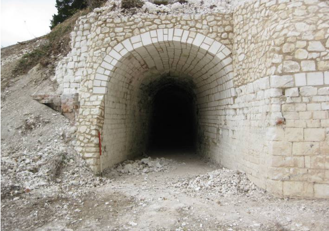
Plate 10 – Westernmost arch of the Grecian Grotto (entrance to tunnel) taken during the current program of reconstruction and consolidation
