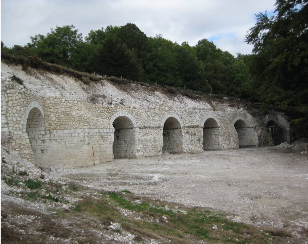
Plate 8 – View of the 6 arches of the Grecian Grotto taken during the current program of reconstruction and consolidation
