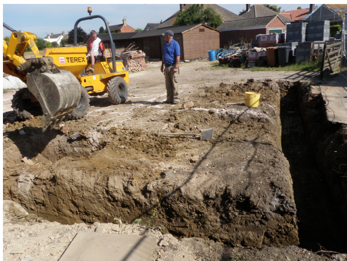
Plate 3 – Excavation of the foundation trenches for the new Holiday lets, looking north
