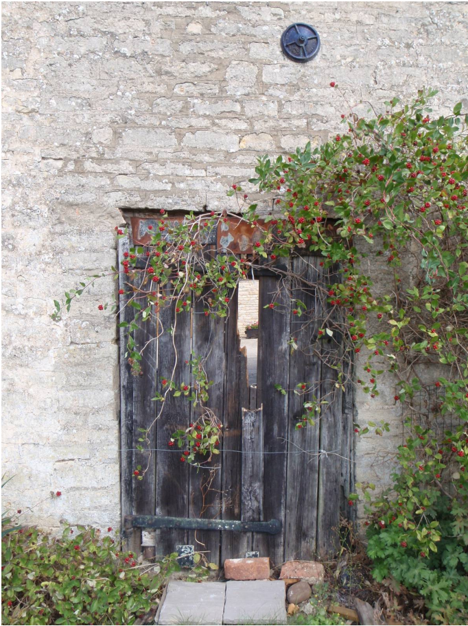
Plate 7 Detail of south elevation of barn showing doorway and cross tie plate, looking north
