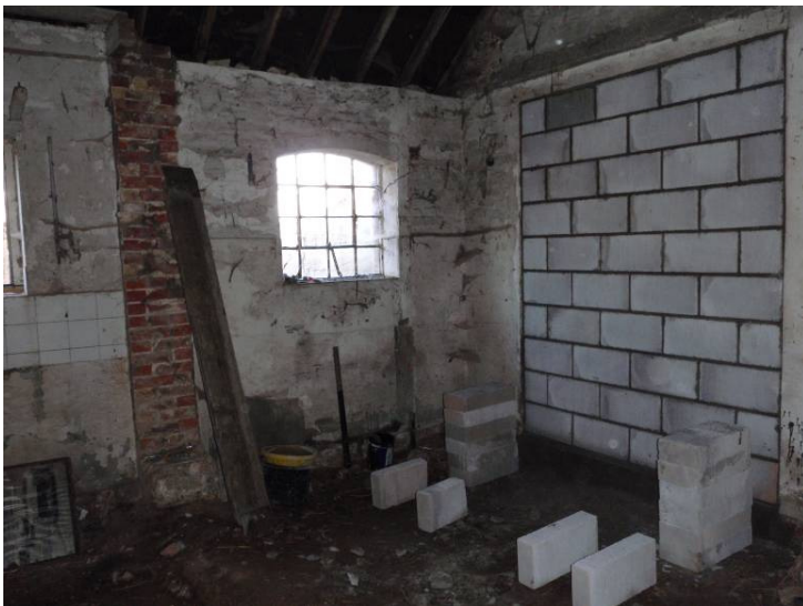
Plate 25 Interior of Range 2, northeasterly room, wall 2b showing blocked doorway and wall 2a showing original window and wall scar, looking north
