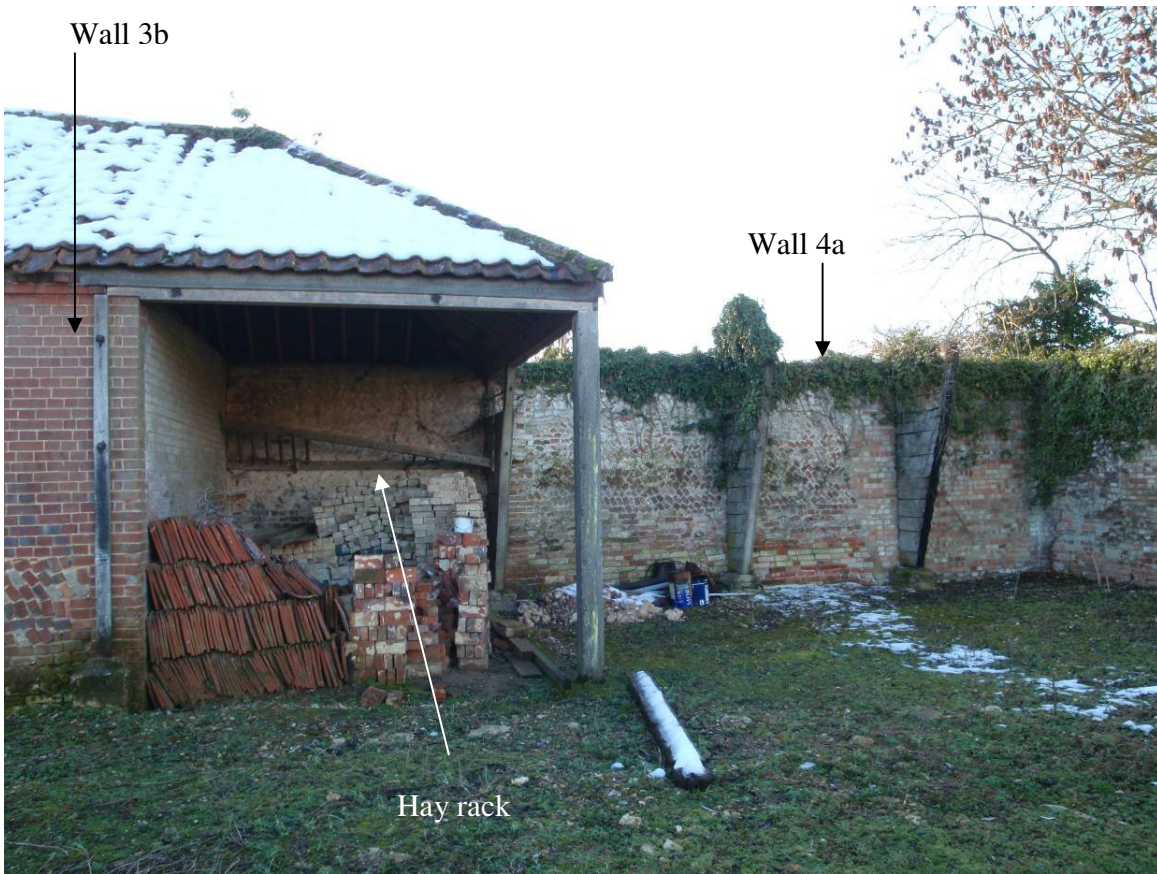
Plate 6 Open-sided shelter wall 3a and hay rack and wooden fixtures of wall 4a, looking southwest
