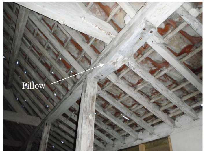
Plate 40 Interior of main room, Range 1, showing change in slope of roofing and retained original wooden pillow, looking east
