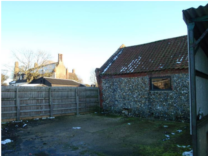
Plate 31 Northern end of Range 1, wall 1a, Abbey Farmhouse visible in background, looking east
