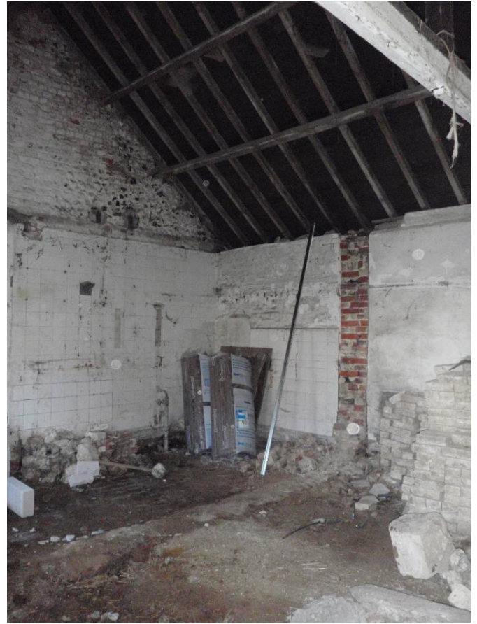
Plate 24 Interior of Range 2, northeasterly room, walls 2b and 2c, showing wall scar across room, looking east
