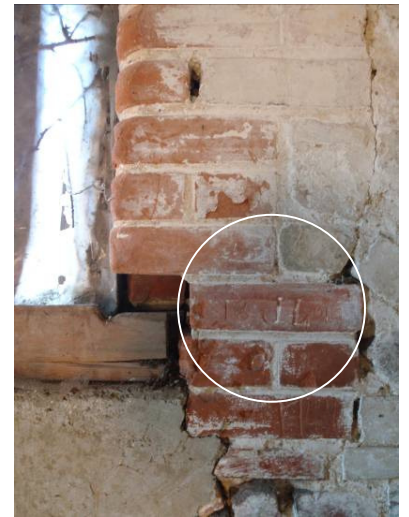
Plate 9 Interior of southern room, Range 3, detail showing graffiti "J L 1801" on brick, looking southeast
