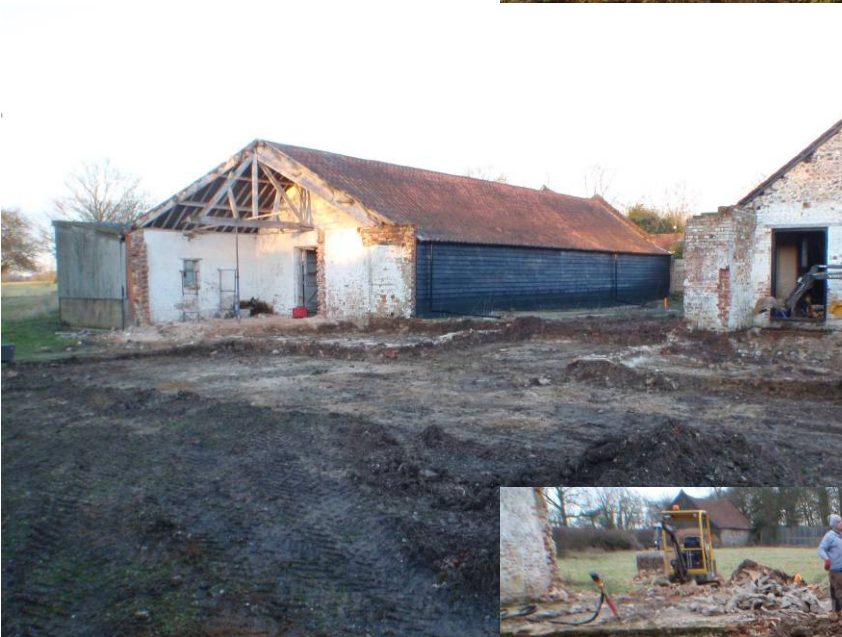
Plate 43 General view of stripped area prior to excavation of wall footings, looking north
