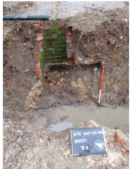
Plate 47 Brick manhole above culvert 041 prior to removal of manhole (see Plate 48), looking southeast
