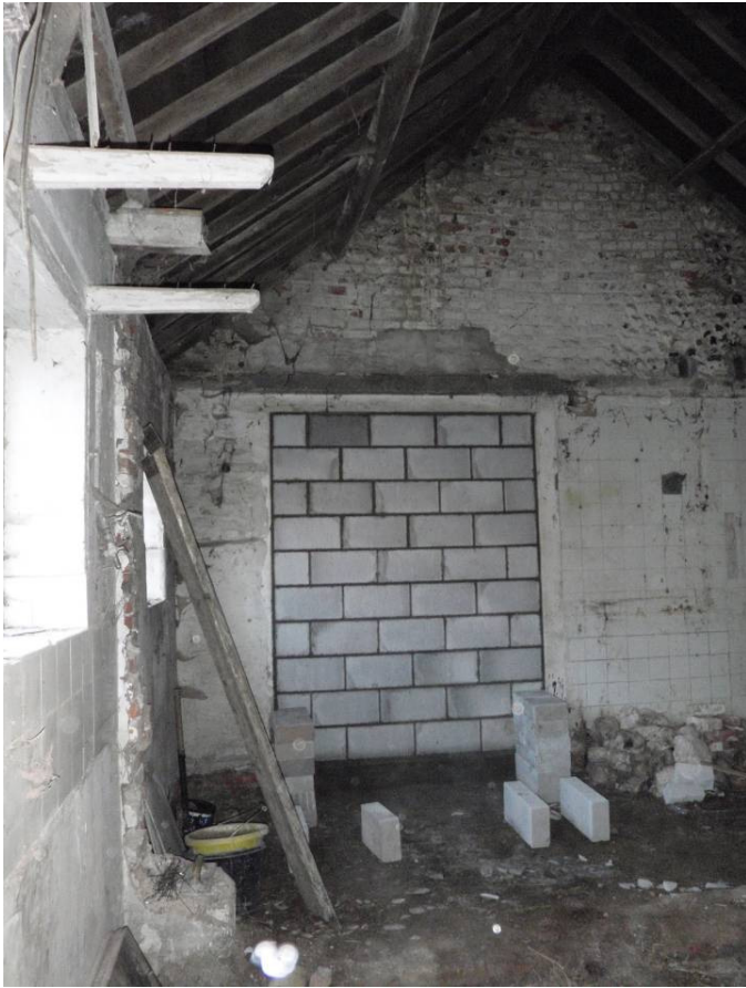
Plate 23 Interior of Range 2, northeasterly room, wall 2b, showing blocked doorway and wooden pegs, possible tack hooks or cistern supports, looking northeast
