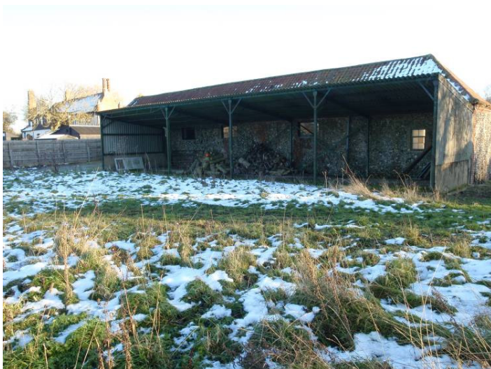
Plate 32 Northwestern wall of Range 1, wall 1a, behind modern lean-to shelter-shed, looking southeast
