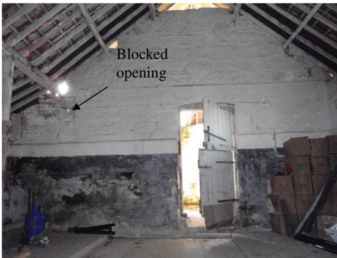
Plate 39 Interior of main room, Range 1, wall 1e showing stable door and blocked opening, looking southwest
