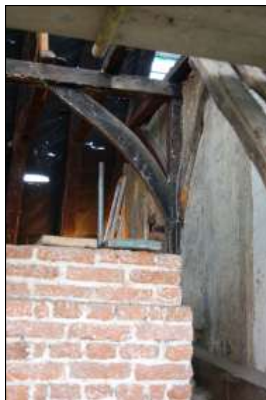
Plate 83: Room F3: crown post
