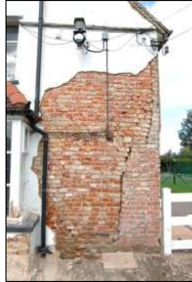
Plate 50: Structural fault in the south wall
