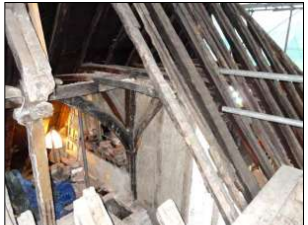
Plate 82: Room F3: crown post
