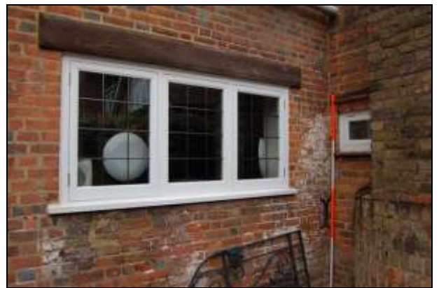
Plate 4: East elevation detail of roof scar.
