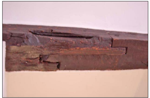
Plate 32: Room F1: counterbladed scarf joint detail
