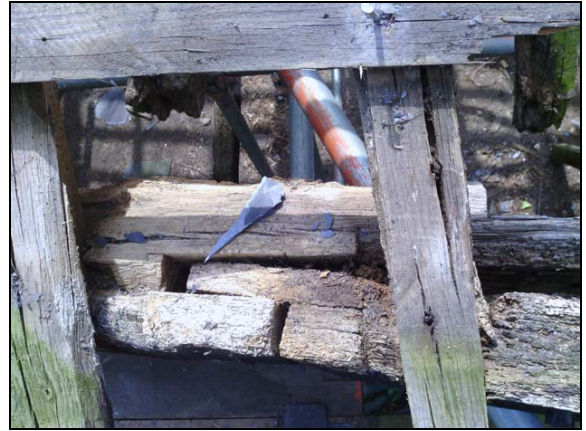
Plate 44: Failed scarf joint in northern wallplate of east barn
