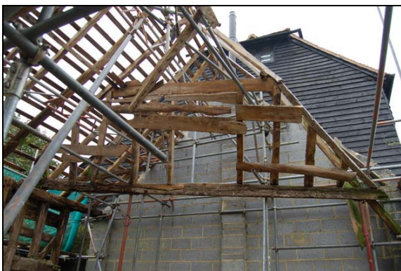
Plate 35: East Barn: remains of west gable end
