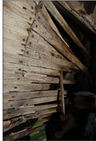
Plate 32: First floor: cut laths on south wall
