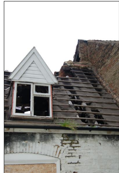
Plate 4: Dormer and chimney remains detail
