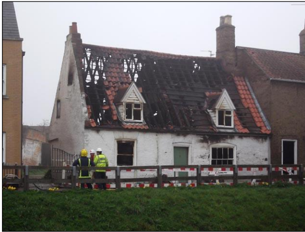
Plate 1: South elevation immediately after the fire (Courtesy of Joan Munn)
