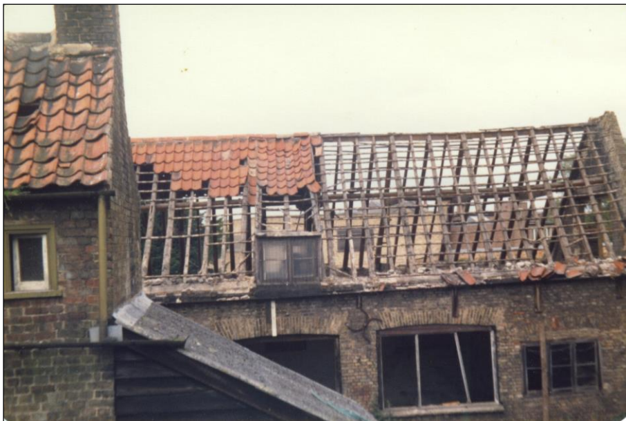
Plate 43: Roof of the former workshop to the north of number 7 (Courtesy of Mel Saxby)
