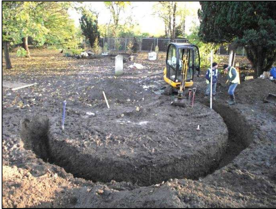
Plate 55: Footing trench for new stone and wood bench in eastern cemetery, looking E
