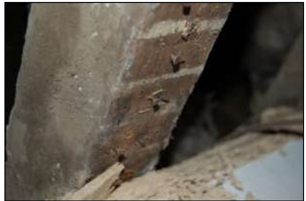
Plate 108: Room F7: modern nails in ceiling joist
