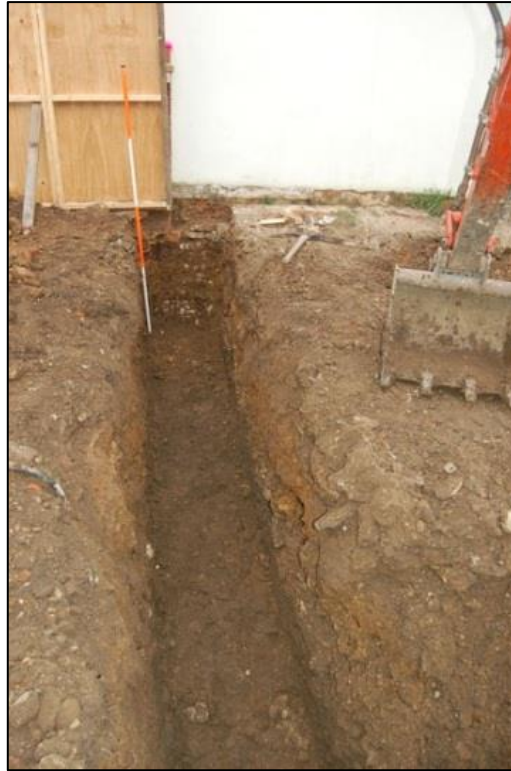
Plate 5: Buried subsoil in southern arm of footing trench, looking north west, 2m scale
