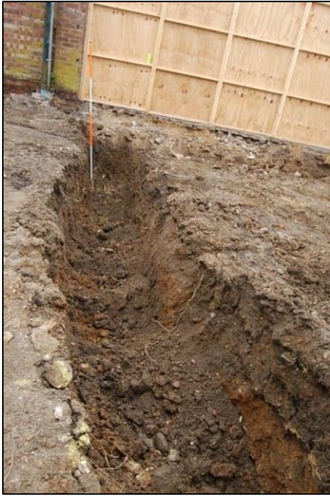
Plate 1: Typical footing trench, showing re-deposited gravel layer, looking south east, 2m scale
