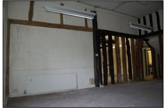
Plate 14: Exposed timbers in western part of Studio 1, looking south
