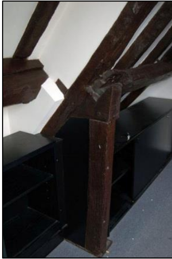
Plate 25: Detail of cut clasped purlin and different roof lines, south side of Office 4, looking south west
