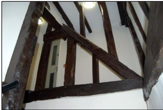
Plate 21: Close studding on external east wall of Archive Store, showing roofline, looking west
