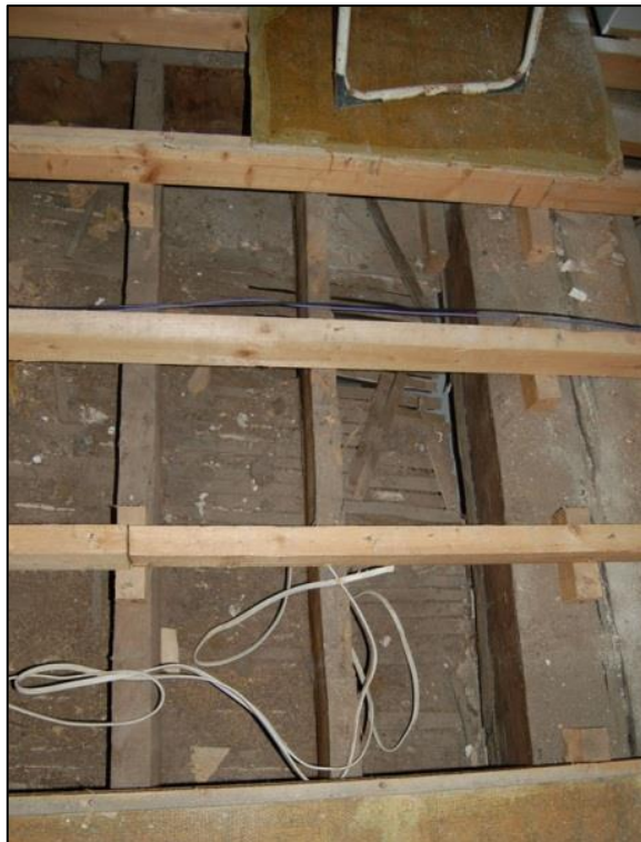
Plate 31: Hole in laths in main bedroom, looking east
