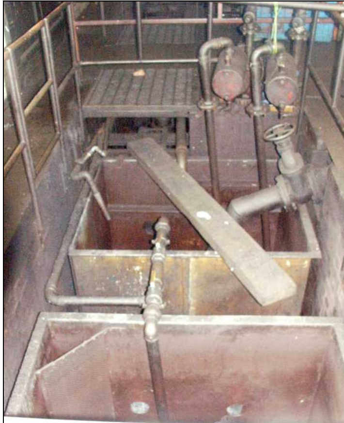
Plate 66: Oil Tanks and Pumps. February 2005
