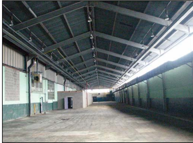
Plate 88: The second southern extension of Building 4, looking east Blocked in windows and cladding of the former south wall visible on the left. Feb 2005
