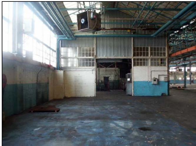
Plate 52: Auto Shop north bay, view towards original east elevation, which latterly formed the west wall of the swarf house. February 2005
