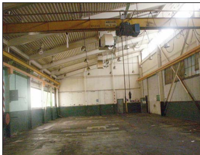
Plate 87: Internal view of the first southern extension of Building 4, looking west. Former external windows visible on wall on right. February 2005
