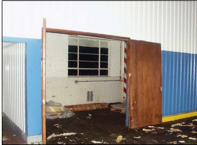
Plate 75: Former external elevation of north wall of the Service Sales Department. Feb 2005
