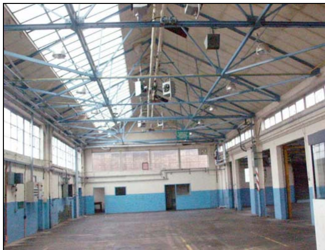
Plate 115: Building 8B internal view looking east Former north wall of Building 8A to right. February 2005
