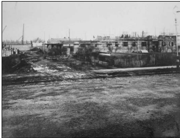
Plate 19: The south façade of Building 2 and the Admin. Block during construction 20 Dec 1941
