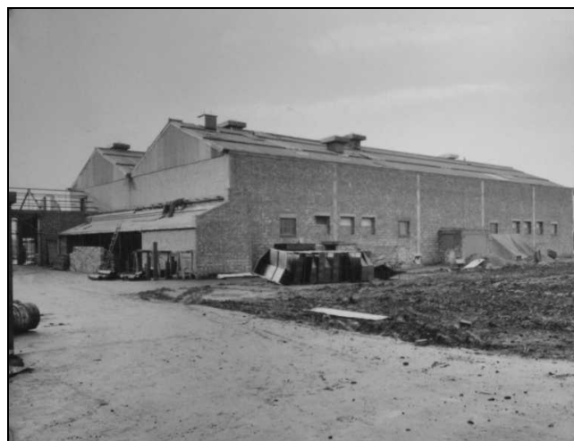
Plate 56: The original north elevation of the Hardening Shop under construction. 8 th December 1942
