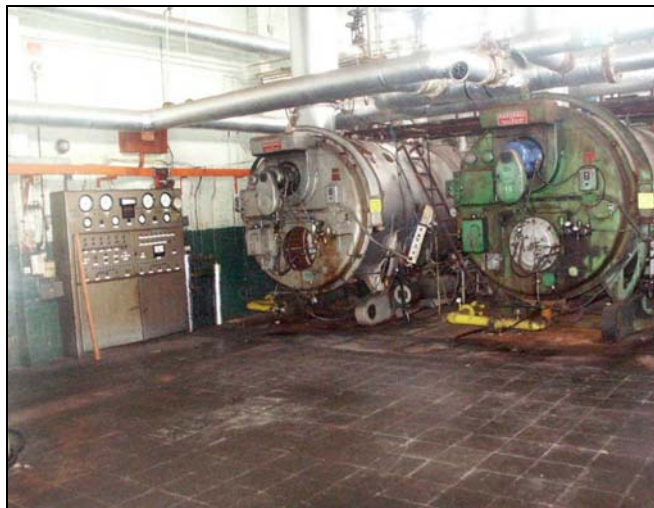
Plate 89: Internal view of the Boiler House, Building 4. February 2005
