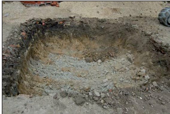
Plate 15: Soakaway to the rear of Plots 7 & 8
