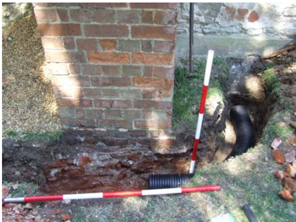
Plate 3: Foundation courses of brick buttress and base of church wall, facing N
