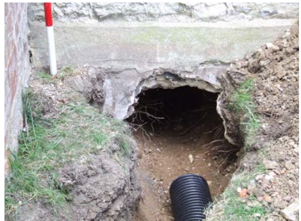
Plate 4: Hole cut through modern concrete at the base of the church wall, facing N
