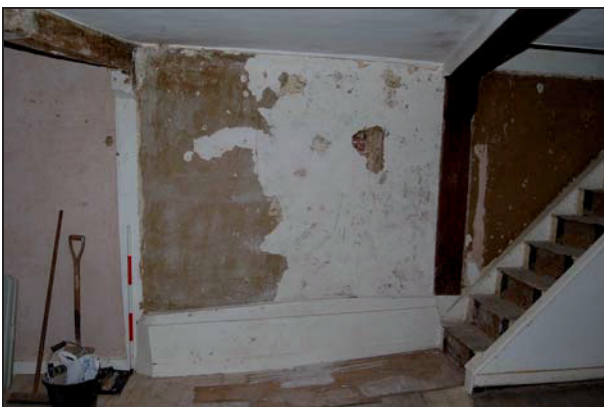
Plate 11: G1: east wall, north of the stairs
