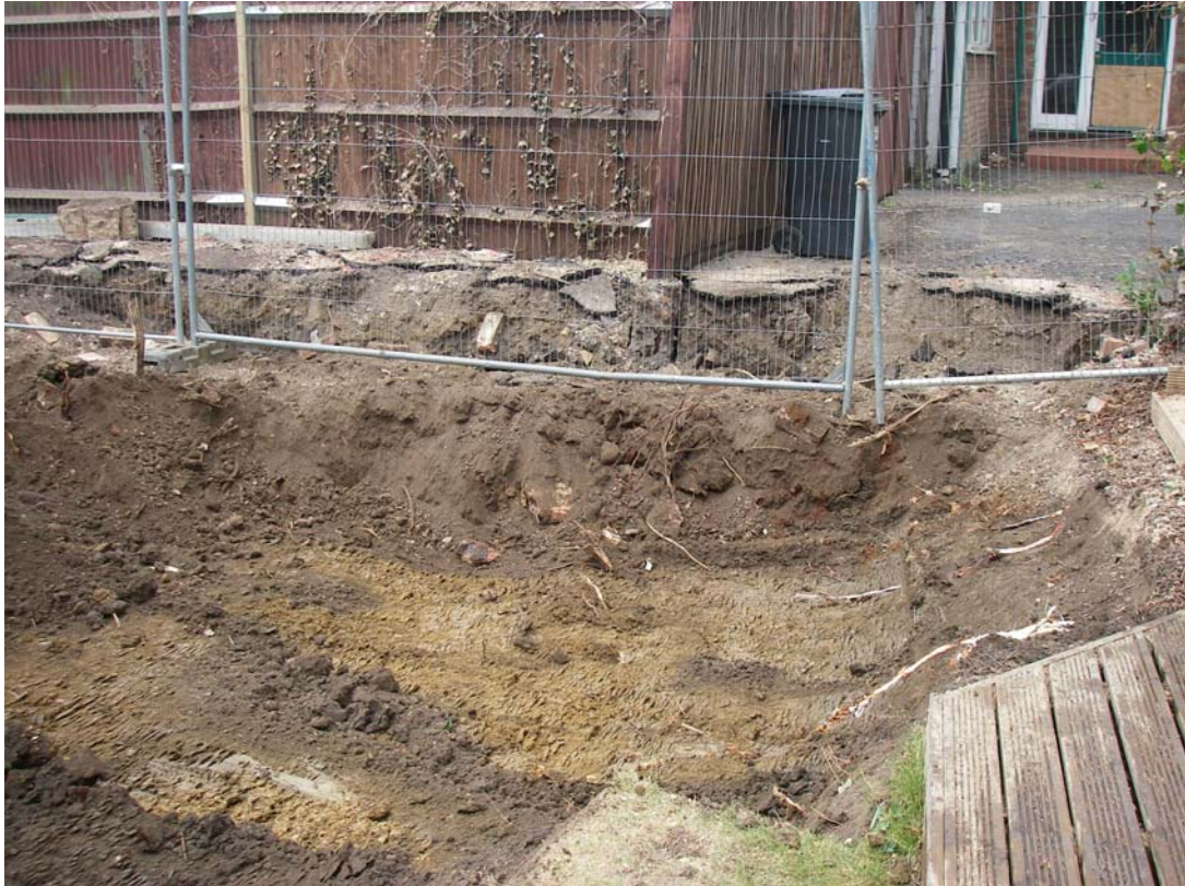
Plate 1: Showing the raised land to the NW where the boundary wall was demolished
