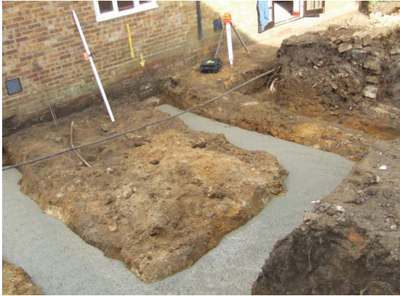
Plate 13: Foundation of northern part of extension with feature [400 ] partly visible at top right, facing NE
