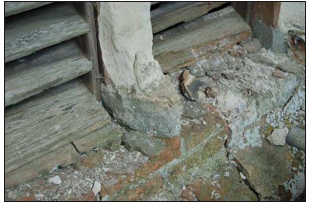
Plate 11: West elevation: Ketton insertion to base of mullion
