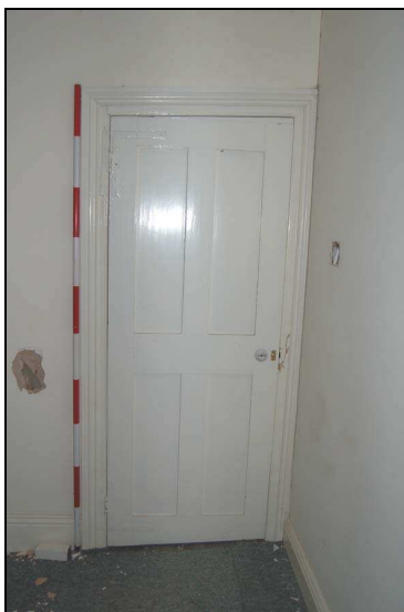
Plate 59: Room F8: 4-panel door with L hinges
