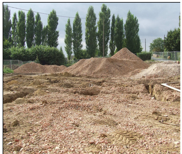
Plate 6: View of the western end of the site and the large amount of bricks from the demolished
