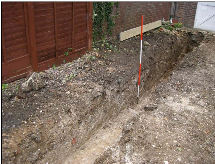
Plate 2: View of western end of foundation trench, looking south west (2m scale)
