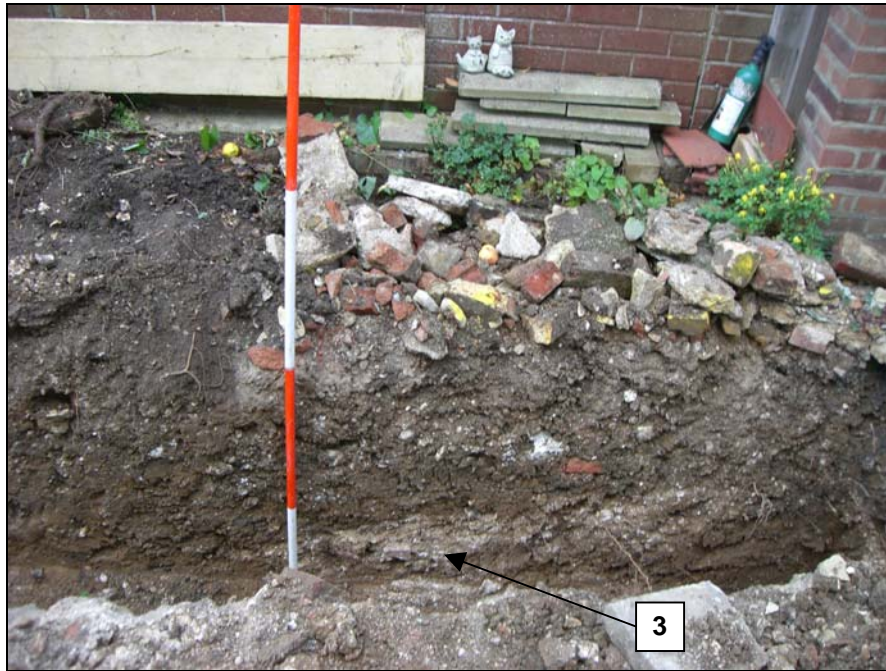
Plate 3: Detail of chalky tip line (3) at western end of foundation trench, looking south (2m scale)
