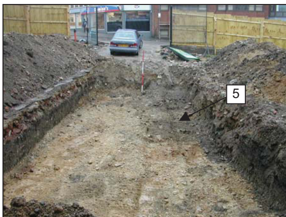
Plate 5: Overall view of trench looking ESE, showing the exposed natural strata (3) and modern disturbance (5) to right (Scale = 2m)
