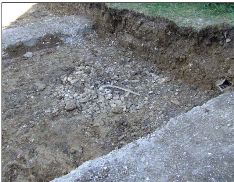
Plate 3: Modern soakaway between Pads 5 & 6
