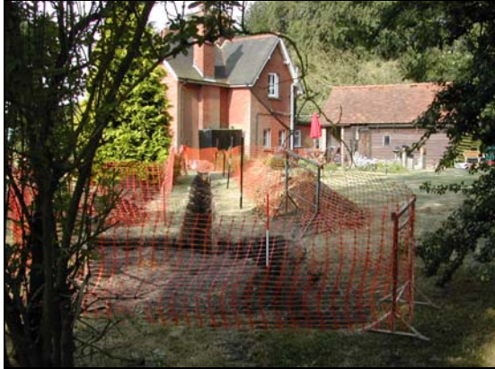
Plate 1: View of service trench between house and Klargester pit, looking west north west , 2m scale 30/06/06
