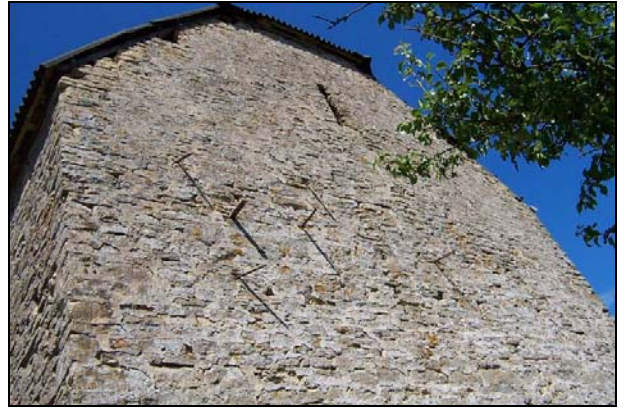
Plate 2: Iron bars in south elevation
