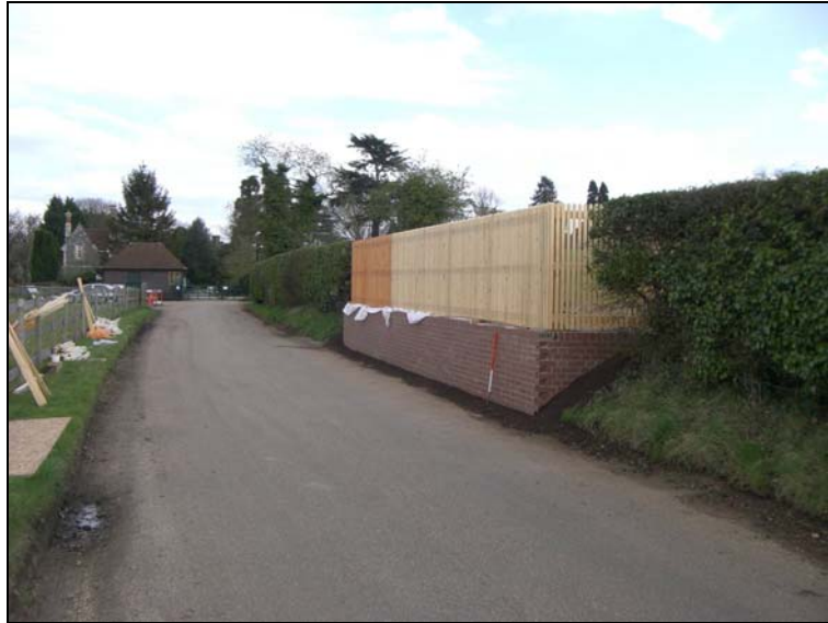
Plate 4: Looking north east to the retaining wall for the new viewing platform
