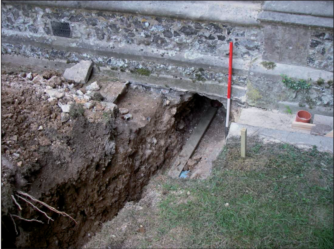
Plate 1: The hole through the north aisle footing
