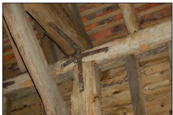
Plate 12: Reversed assembly and iron ties on Truss 3
