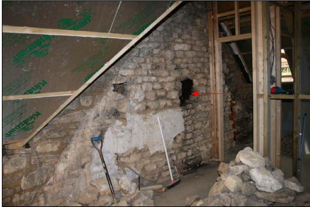
Plate 1: East wall (the arrow marks the location of the soot lined cavity)
