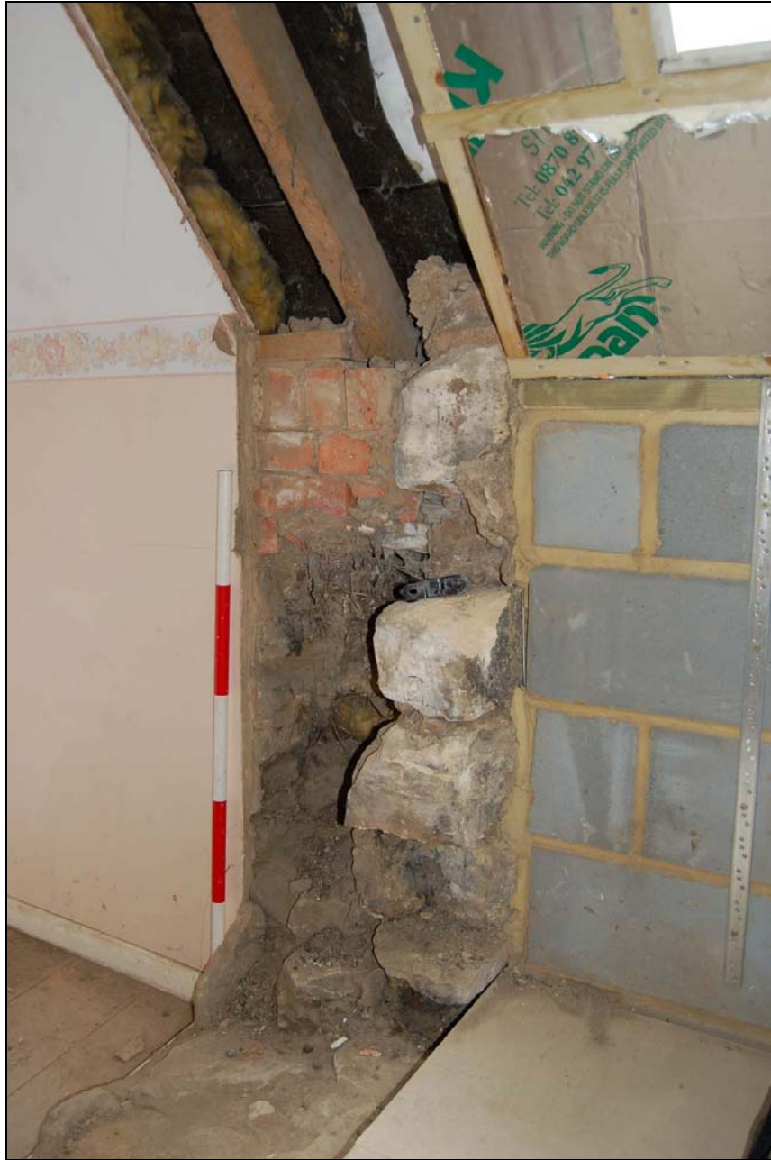
Plate 3: North wall showing the modern rafters and brickwork to the left of the new extension
