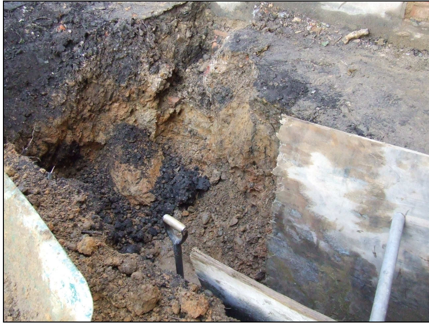
Plate 3: Collapsed trench, looking northwest
