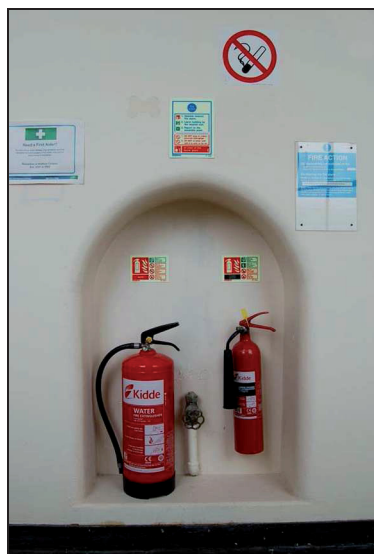
Plate 156: Detail of fire extinguishers in arch on second floor
