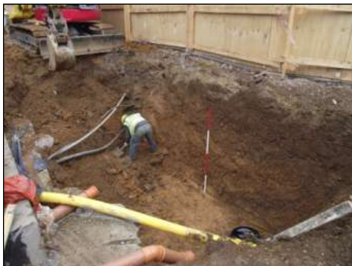
Plate 3: Extension A: soakaway
