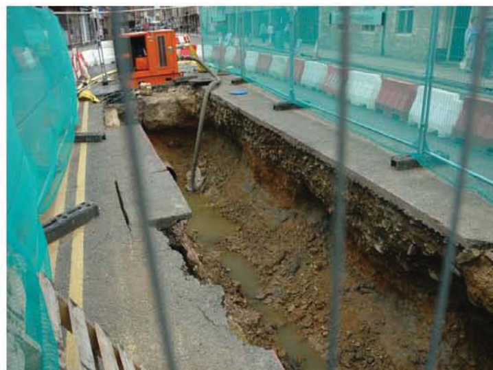
Plate 6: Trench west of Lincoln Road revealing earlier surfaces (almshouse visible top right).
